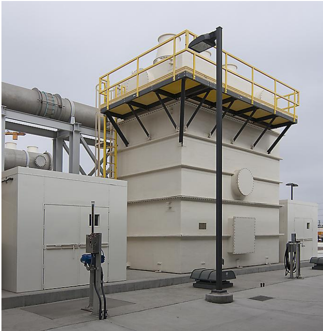
Decarbonator (CO 2 Stripping)
