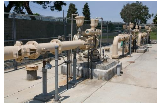
Typical injection well - OCWD
